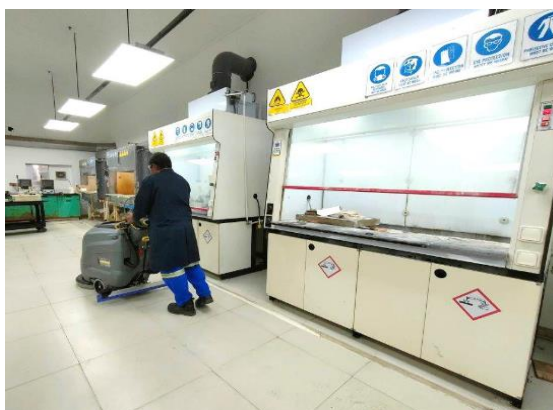
Picture. 4. New Design on Fume Hood and Flooring.
