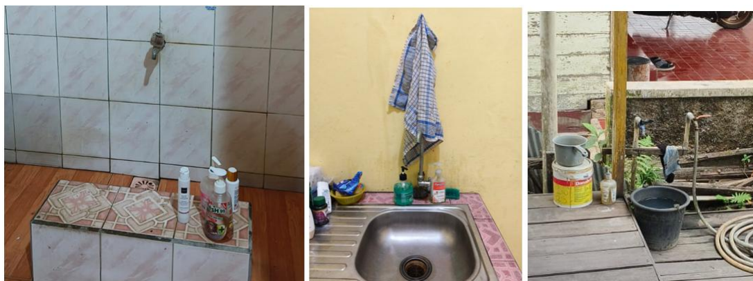
Figure 1. Condition of Handwashing Facilities
